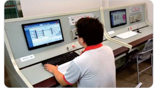
Control room & Graphical HMI
